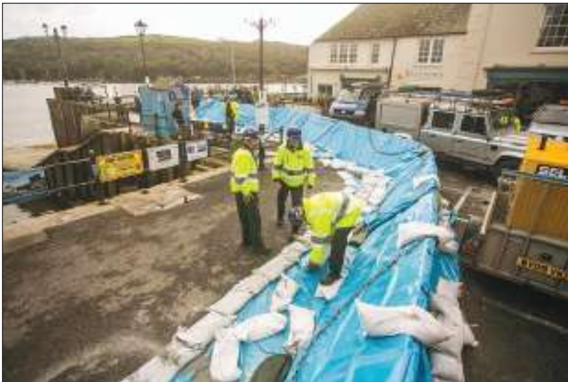
Flood defences were erected in Fowey, Cornwall
